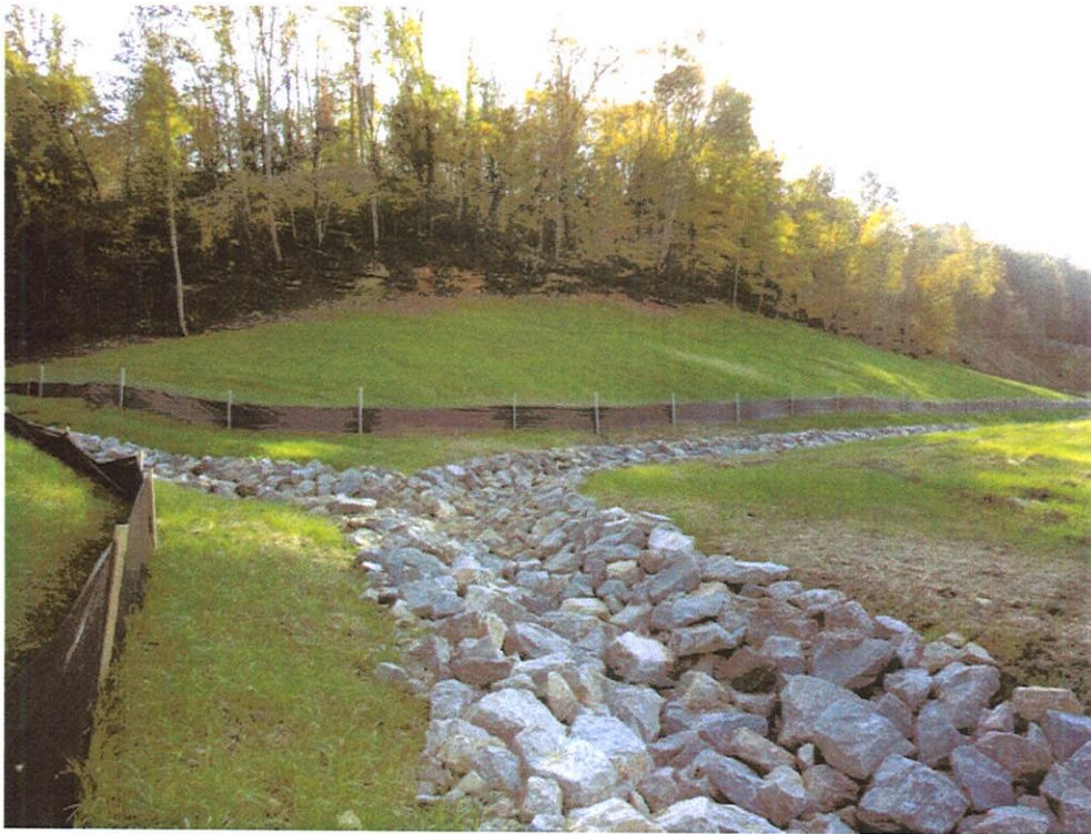
Prospect Valley Highwall #4 – DEP14433
