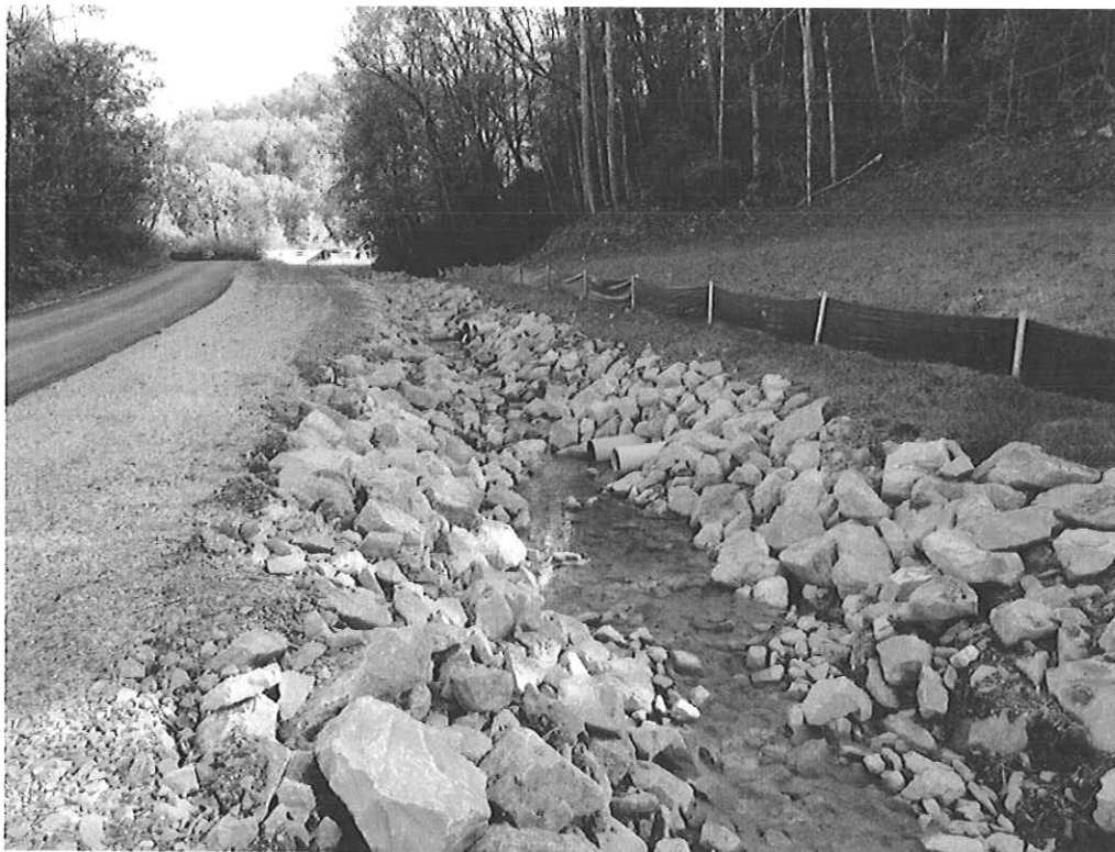
Prospect Valley Highwall #4 – DEP14433
