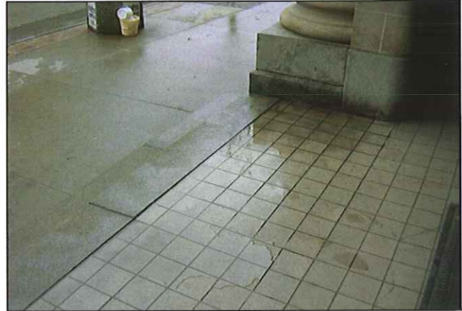
Ponding water travels into basement due to lack of waterproofing beneath entry
