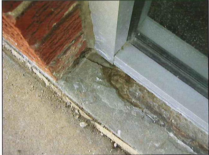
Deteriorated sill stone causes water infiltration
