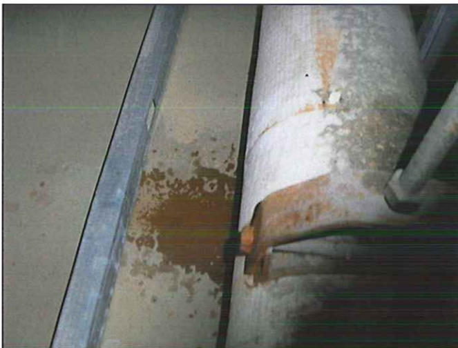
Leakage showing up on steel below in the basement area
