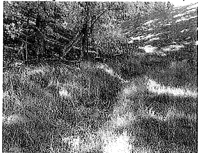
Photo No. 4: Right groin seepage area.
