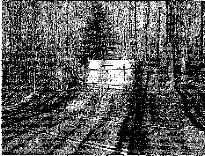
150 GPM Water Booster Station Located in Audra State Park Phase II
