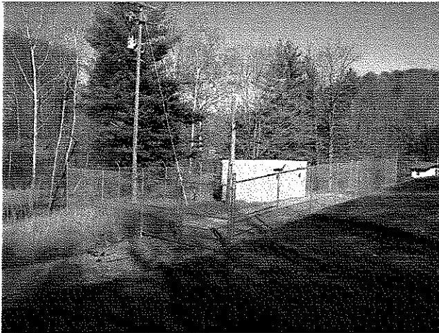
50 GPM Wilsontown Booster Station
