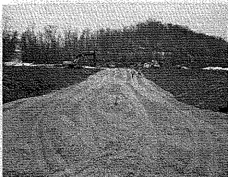
Entrance Road Construction at Kulseth Industrial Park, outside of Fairmont, West Virginia. Kulseth was one of three industrial parks engineered by Thrasher for the Marion Regional Development Council
