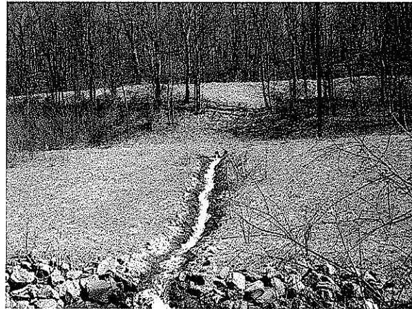
Wet mine seal with rip rap channel
