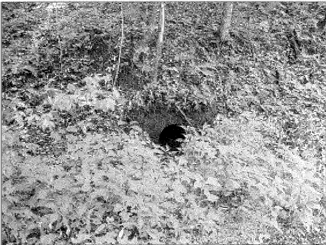
PHOTO NO. 4 - CULVERT CONVEYING MINE DISCHARGE TO DITCH ALONG LOOP BRANCH ROAD
