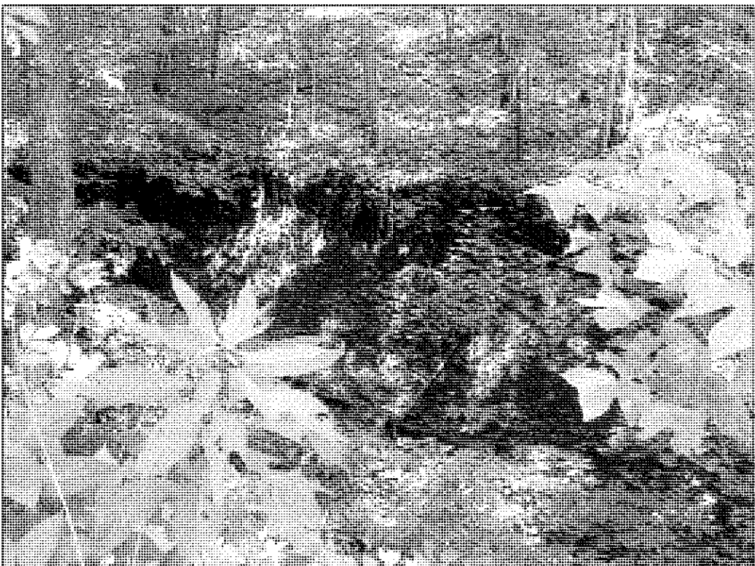
PHOTO NO. 6 - UNDERCUTTING AT TOE OF REFUSE PILE ALONG CREEK
