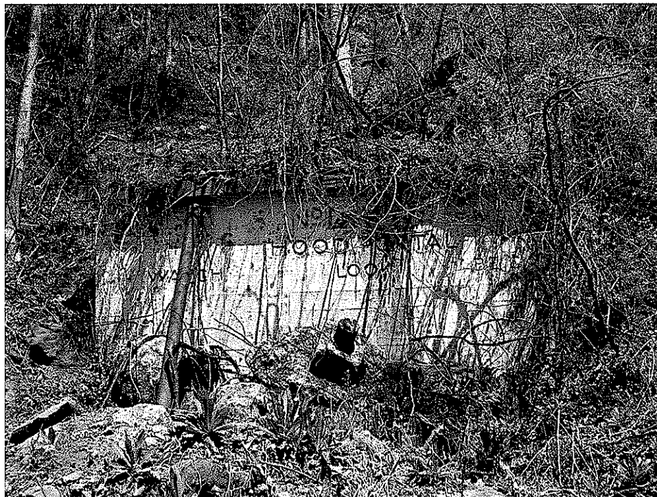
Picture 4 shows a cracked Hood Portal seal.
