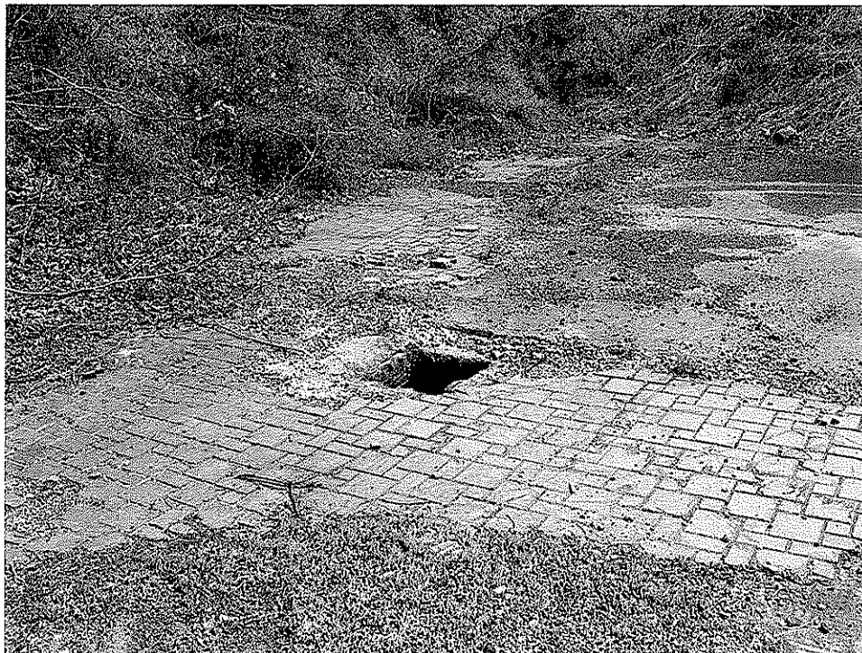
Picture 8 shows a hazardous access hatch.
