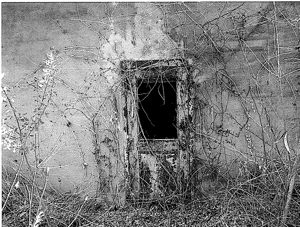
Picture 6 shows an unobstructed entrance to a hazardous area of the prep plant ruins.
