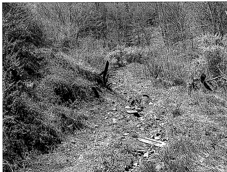
Picture 3 shows an eroded area of one of the dangerous piles and embankments.
