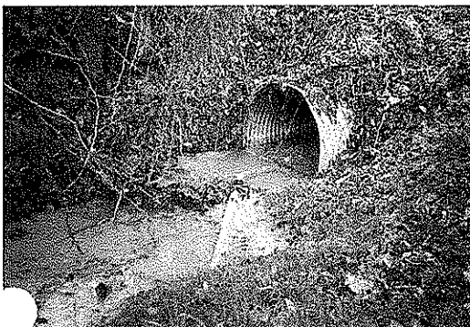
Outlet pipe before remediation
