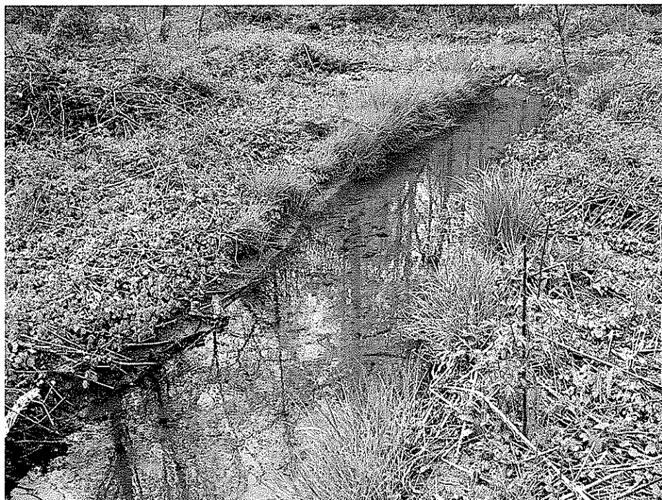
Picture 2 shows storm water after escaping from the breach.
