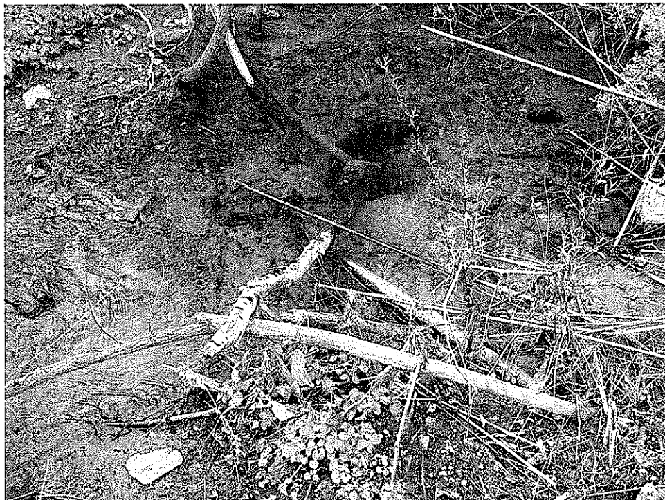
Picture 1 is of a breach in the drainage system where water returns to the surface.
