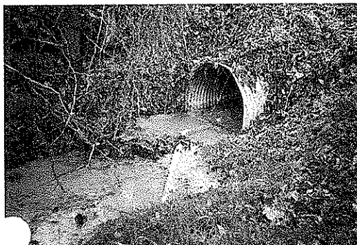
Outlet pipe before remediation
