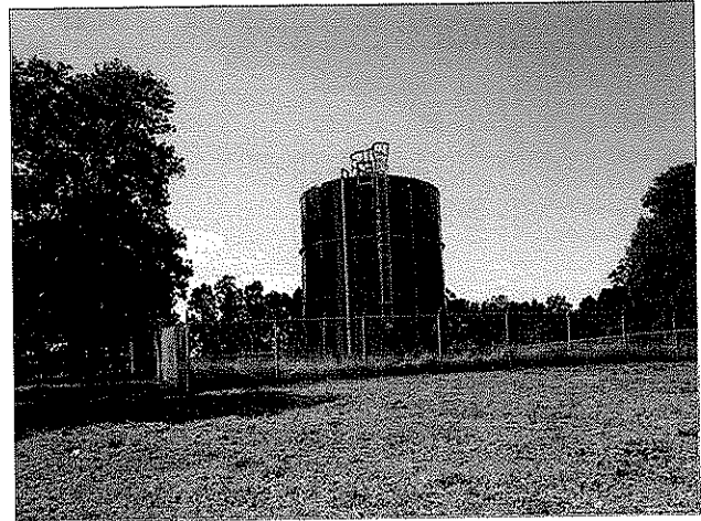
105,000 Gallon Water Storage Tank on Tallmansville Road Near Mt. Carmel Church Road
