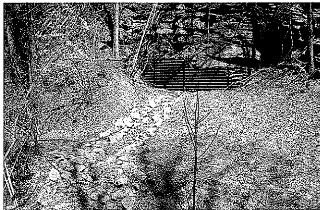
Bat Gate with rip rap channel
