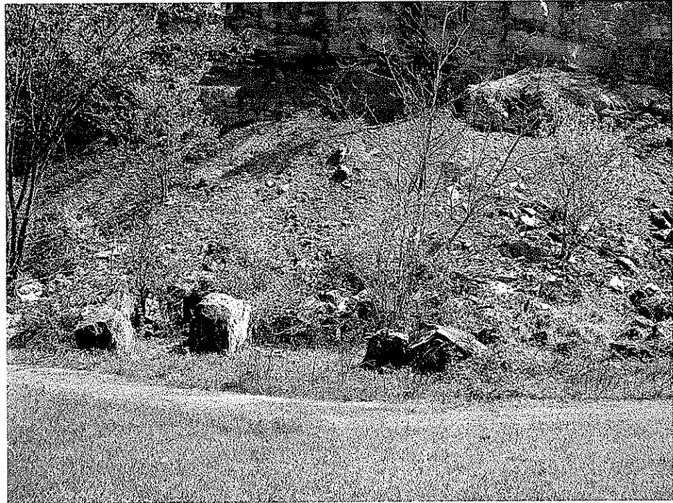
Picture 4 shows the accumulation of eroded material at the base of the highwall.
