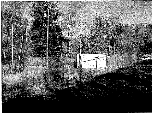
50 GPM Wilsontown Booster Station
