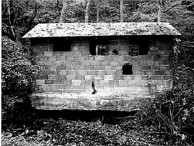
Figure 2—Concrete Block Structure. The stream has undermined the structure's foundation. The structure may collapse into the stream and cause flooding.
