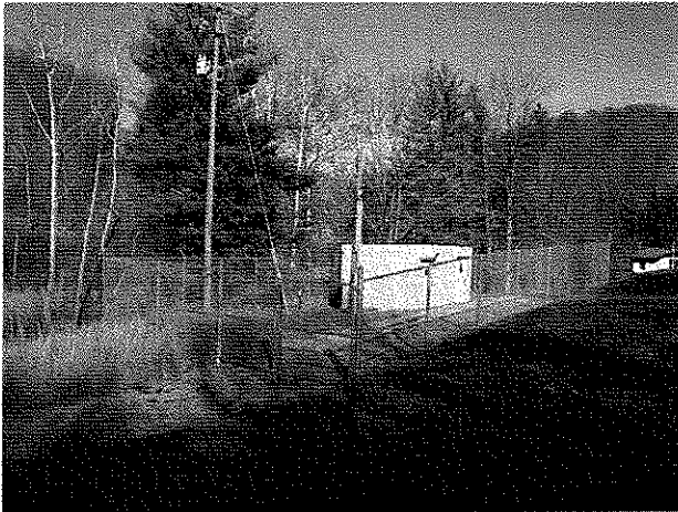
50 GPM Wilsons town Booster Station
