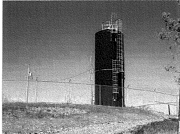
43,000 Gallon Salem Ridge Water Storage Tank
