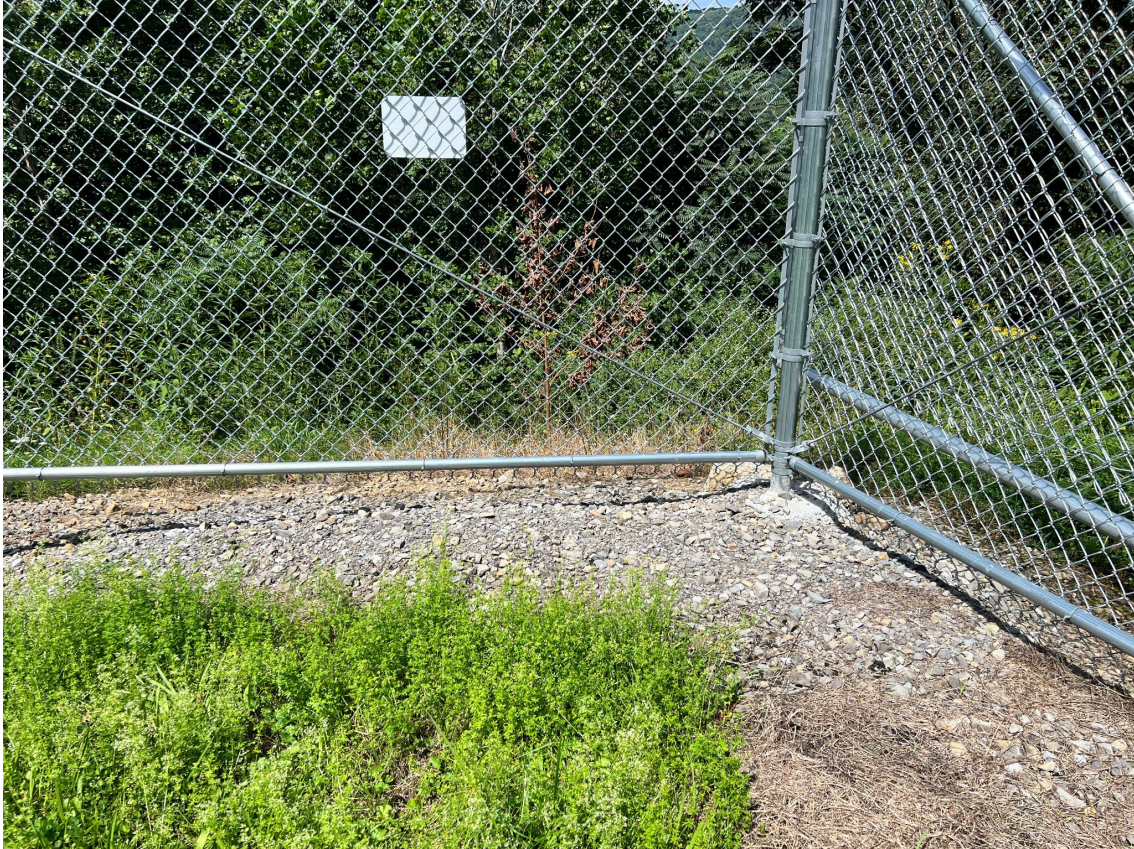
Fence corner / braced gate-post condition and uneven rock subgrade representative of localized forming challenges.
