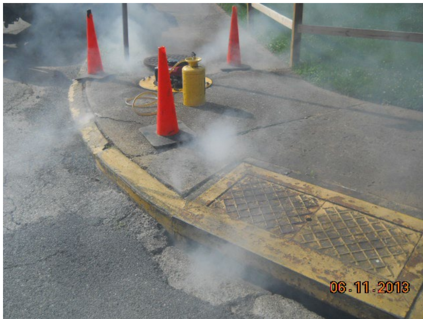
Smoke Test, Downtown Glenville
