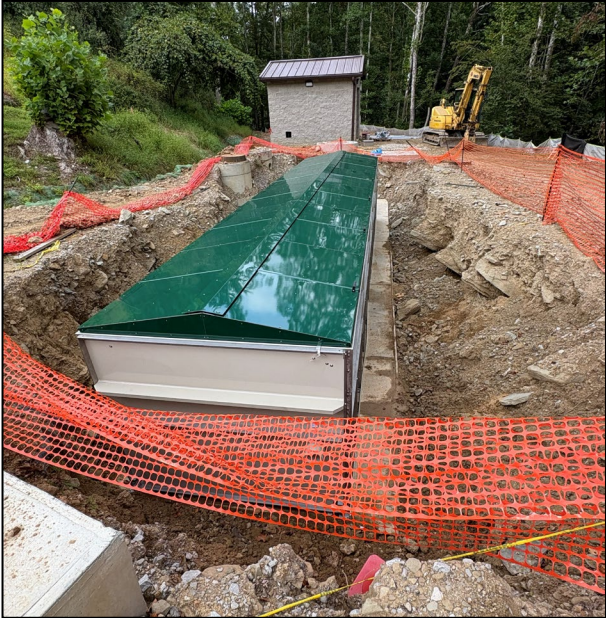
RBC unit with tertiary treatment (filter) building in the background.
