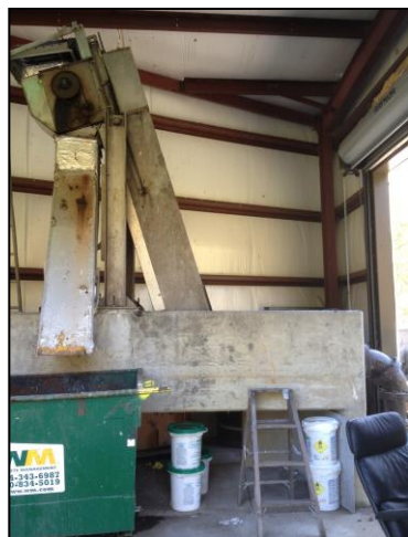
Mechanical Bar Screen to be Replaced
