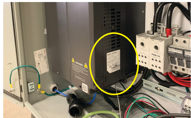
Dura Impulse GS4 Module 2: Located on the side of the unit inside the control panel box.
