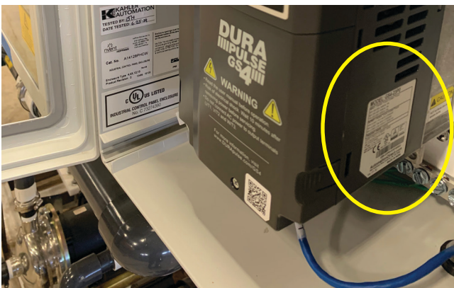
Dura Impulse GS4 Automation Direct: Located on the side of the unit inside the control panel box.
