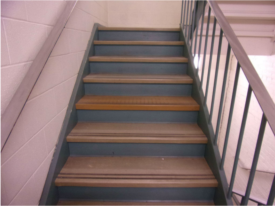
PHOTO 7 North Stair Photo Of Stair Treads To Be Replaced
