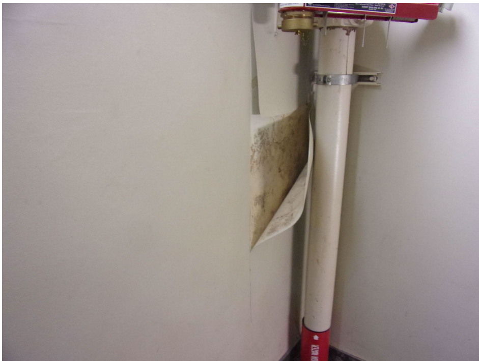
PHOTO 6 South Stair Photo Of Peeling Wall Covering
