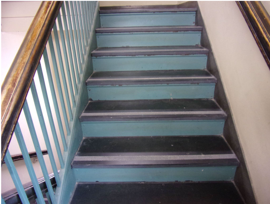
PHOTO 5 South Stair Photo Of Stair Treads To Be Cleaned
