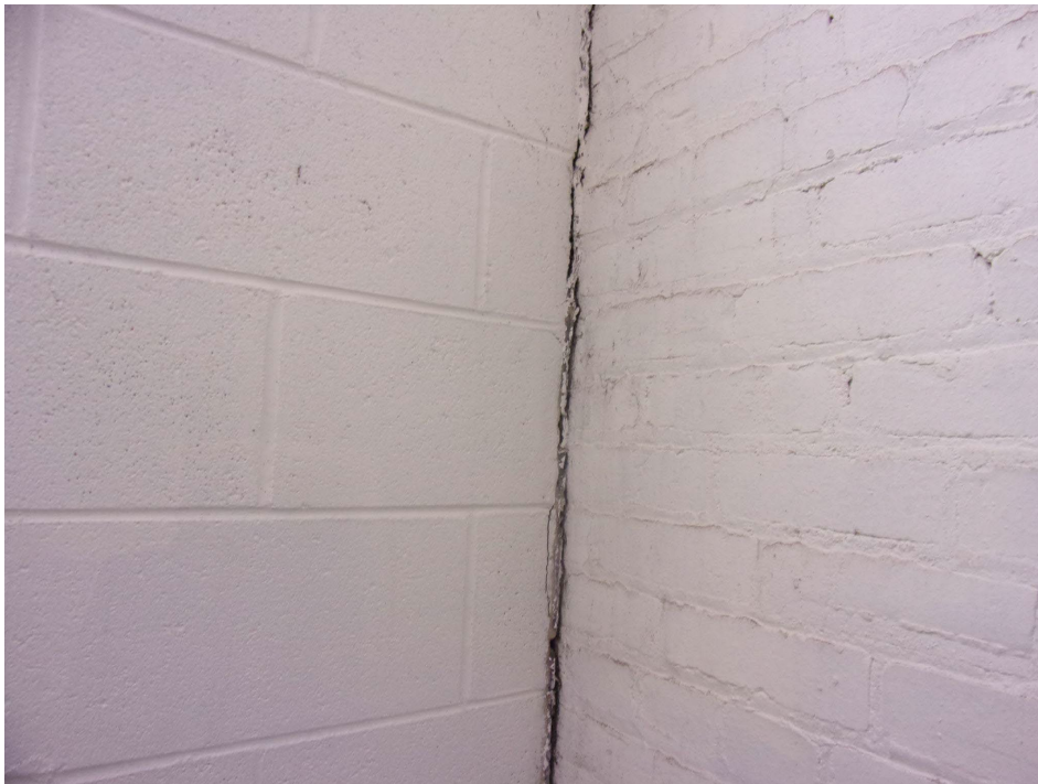
PHOTO 12 North Stair Photo Of Crack To Be Caulked
