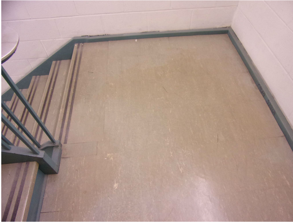
PHOTO 11 North Stair Photo Of Tile Landings To Be Replaced
