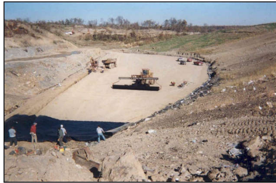
Construction of the 60-mil HDPE geomembrane over the prepared soil subgrade and excavation of perimeter anchor trenches.
