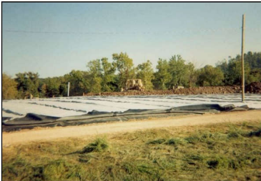
Placement of the final soil cover layer over the geosynthetic layers of the cap.
