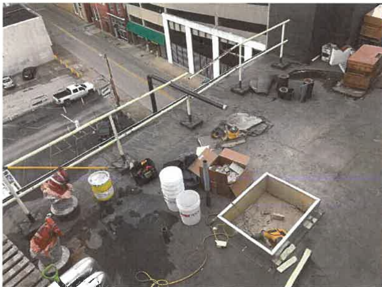
Contractor is making penetration thru the roof for ductwork.
