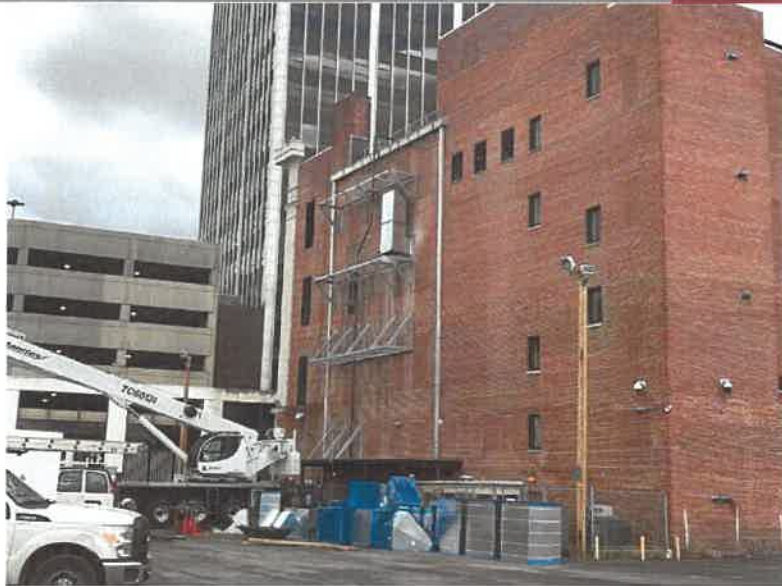
Back of the building with new steel supports and ductwork installation has started.
