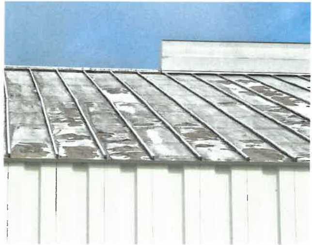
Pieces of the hangar elastomeric coating have detached from the roof deck.
