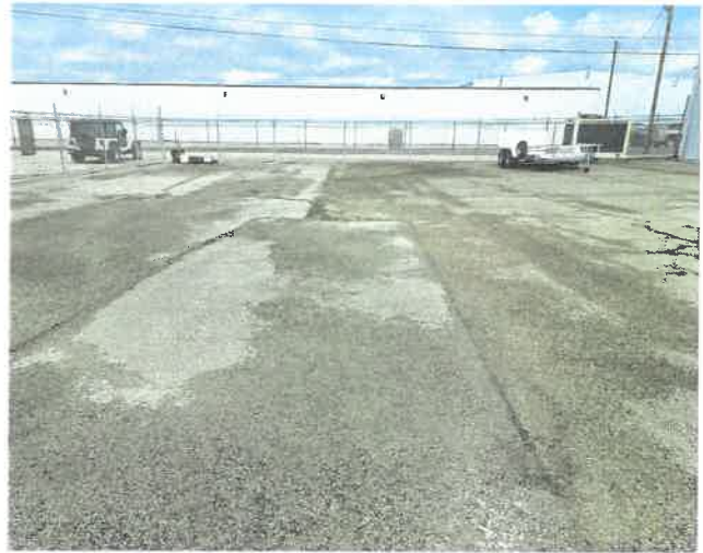
Existing pavements can be milled and overlaid to improve drainage to existing inlets.
