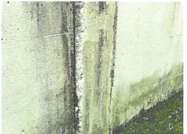
The masonry deterioration of the hangar walls does not appear to be structural in nature and repairs should be relatively simple.
