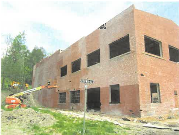
Masonry repair and cleaning on the Coal Heritage Discovery Center in Mt. Hope.
