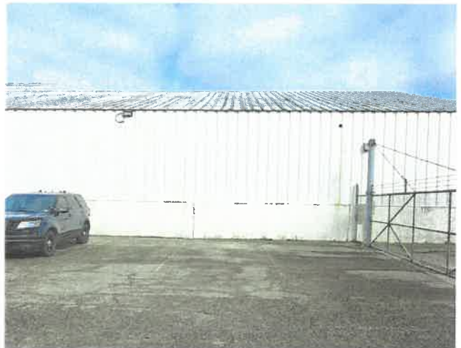
The hangar wall panels appear to be in good condition, with only normal wear and tear. Cleaning and painting should extend the life of the panels.
