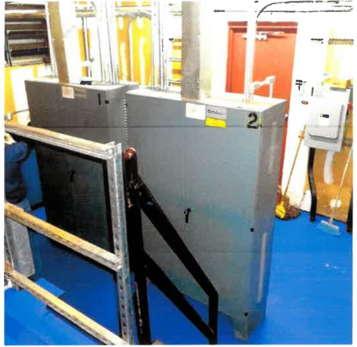
Machine Room After Modernization
