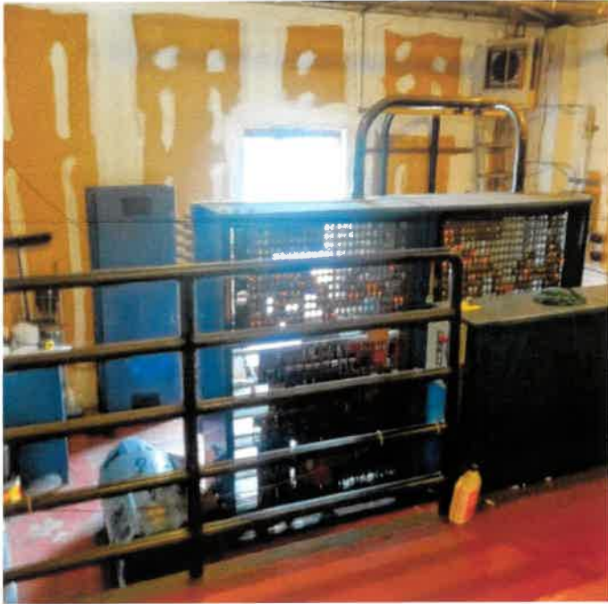
Machine Room Before Modernization
