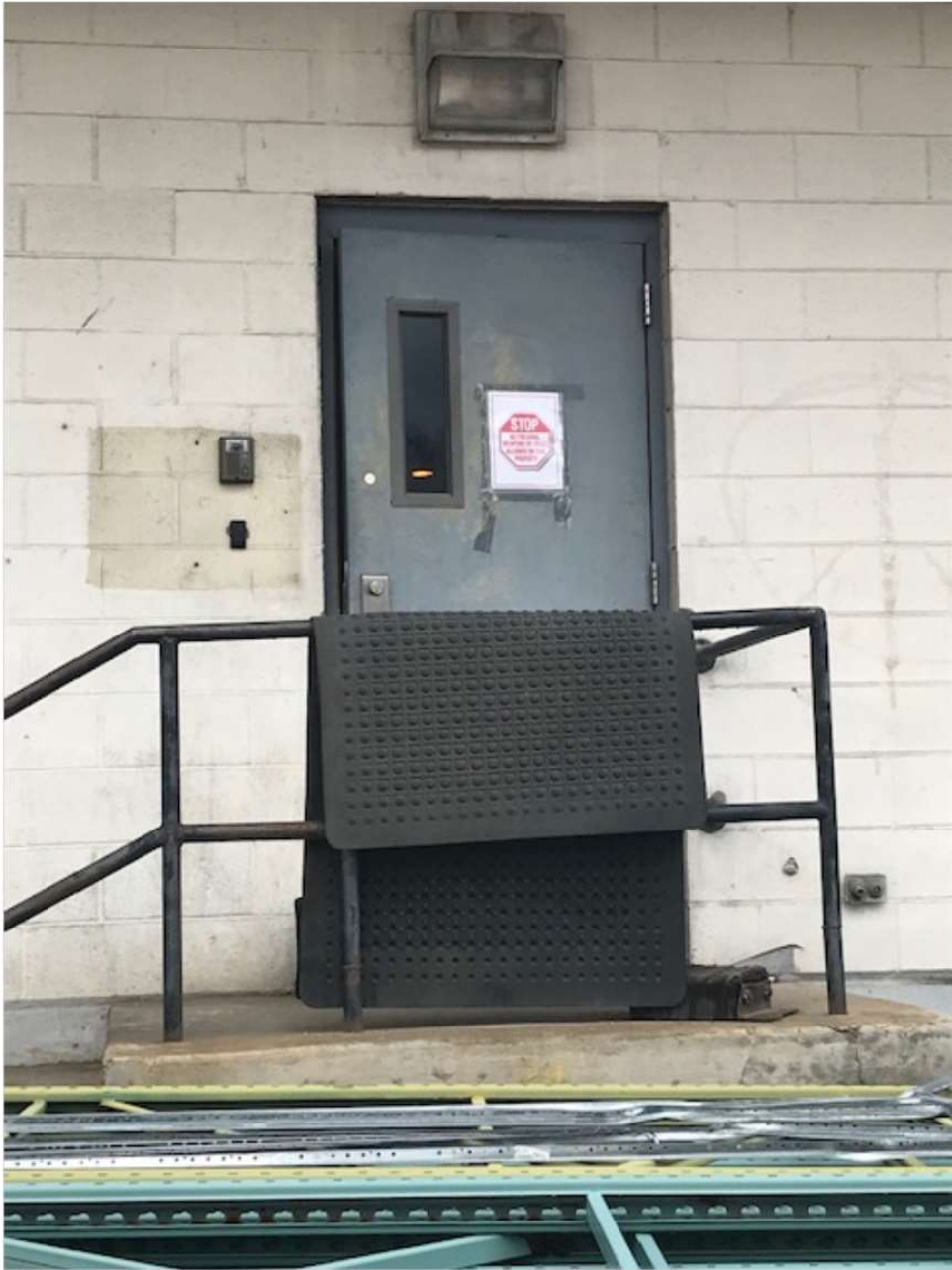
Left Side Door Existing Equipment Photo 1
