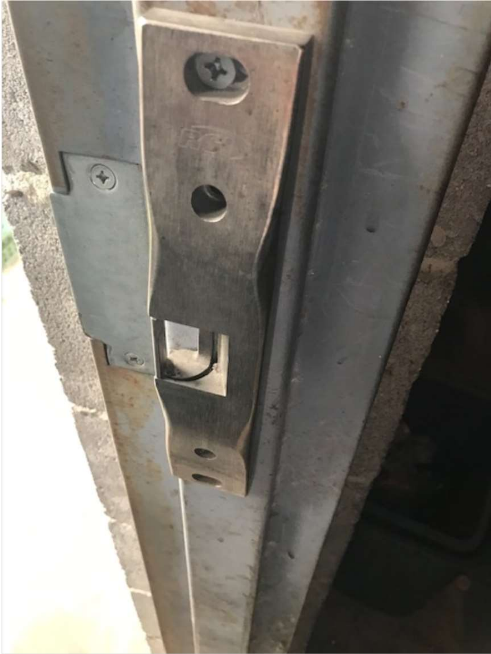
Left Side Door Existing Equipment Photo 2
