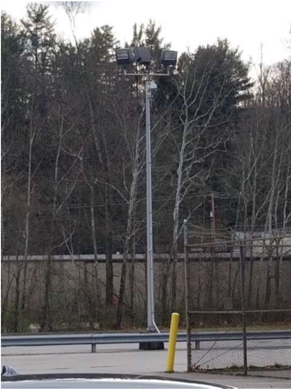
CCTV Outdoor Camera Locations (Parking Lot Light Pole) To Be Removed
