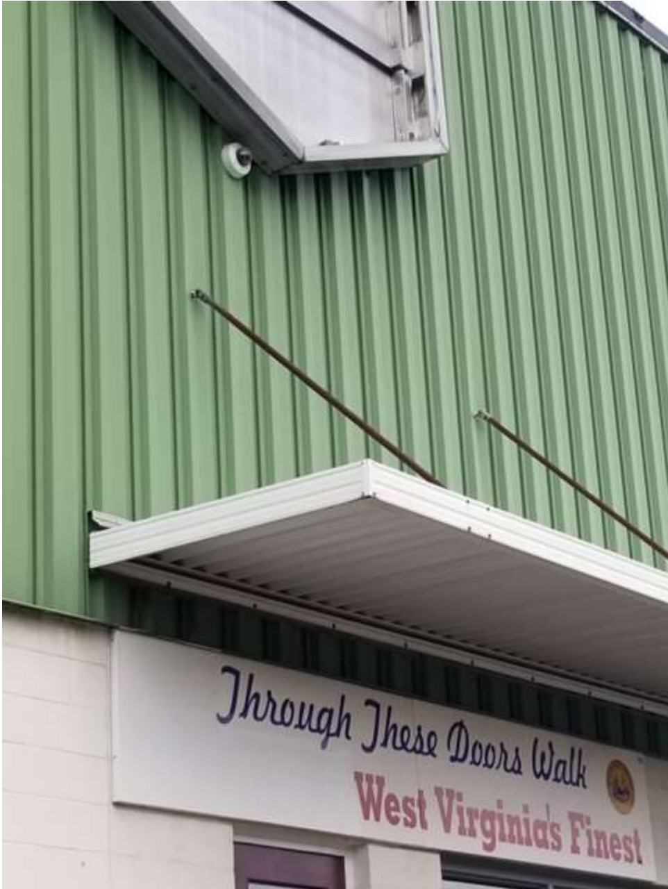
CCTV Outdoor Camera Locations (Main Entrance Location)
