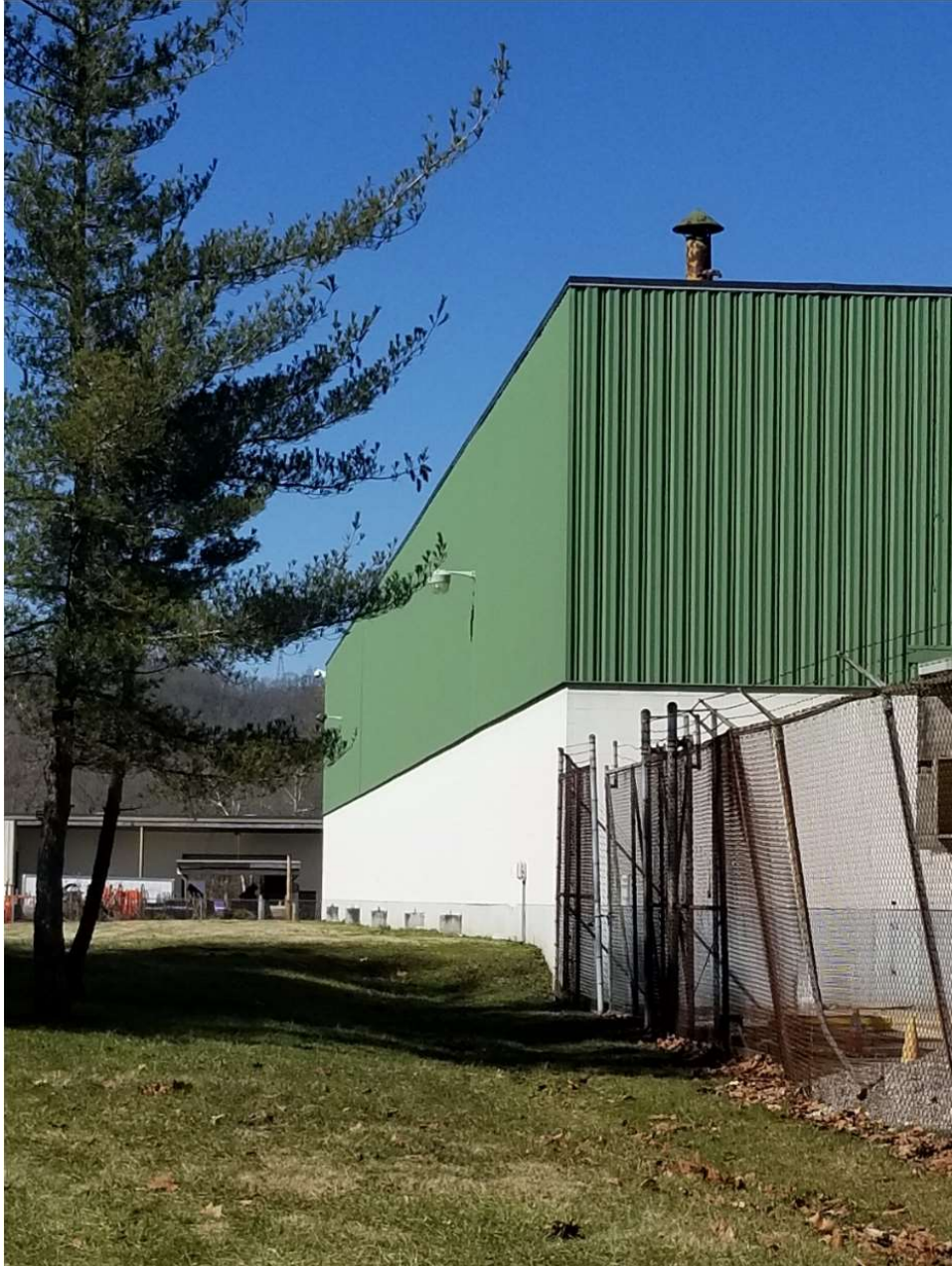
CCTV Outdoor Camera Location (Left Side View from Front of Building)
