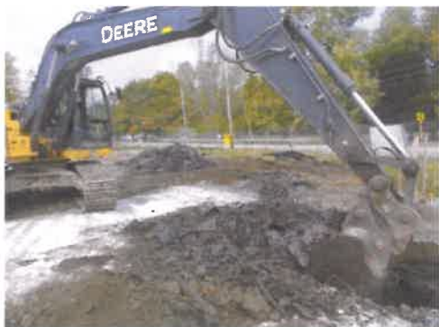
Rubber Dump encountered at North Reservoir Dam
