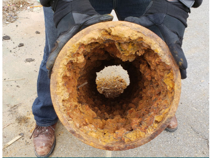
Corroded Water Pipe National Institutes of Health
