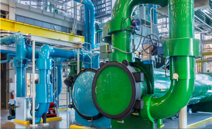
District Energy Facility Chillers Harvard University
