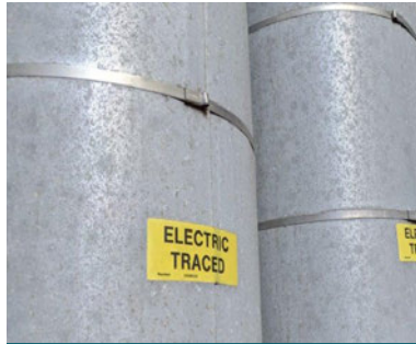
Freeze Prevention is an important design element for cold climate operation
