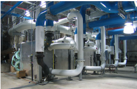
US Capitol Power Plant Free Cooling Heat Exchangers (10,000 Tons) / Architect of the Capitol
