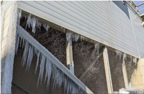
Prevention of cooling tower icing is a key design consideration for safe free cooling operation
