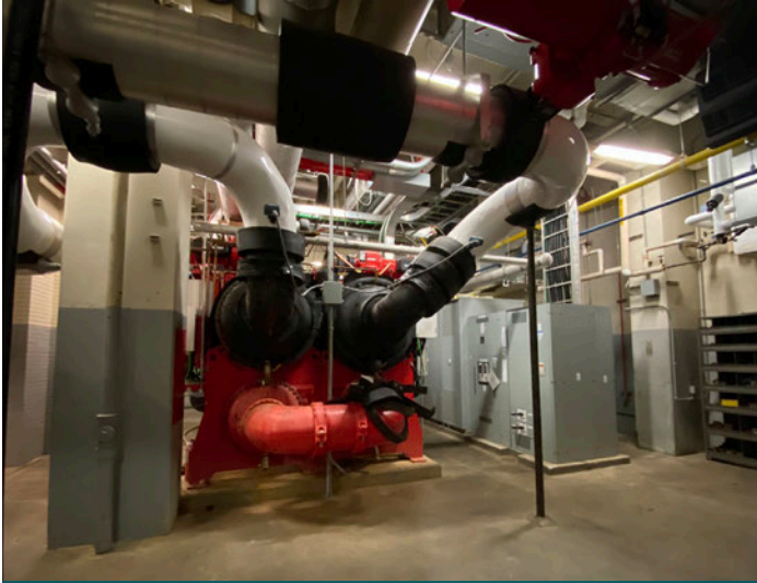
Chiller at the East Campus Utility Plant University of Cincinnati
