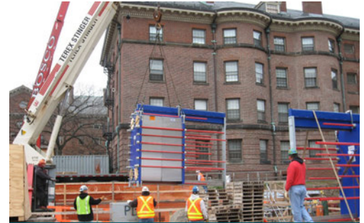
Free Cooling System Installation (3,000 Tons) Harvard University
