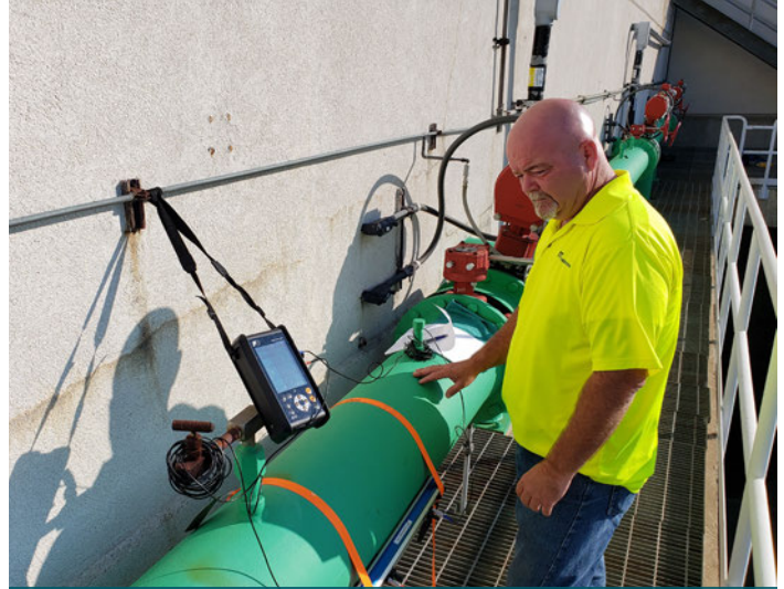
Cooling Tower Testing, Ronald Reagan Washington National Airport Metropolitan Washington Airports Authority
