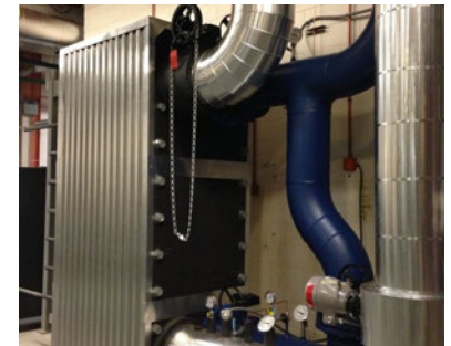
Free Cooling System (1,700 Tons) Georgia Tech
