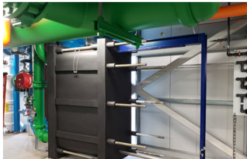
Free Cooling System (500 Tons) University of Massachusetts Amherst
