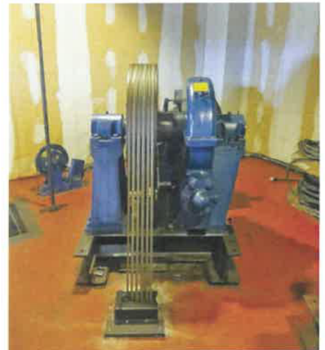
Outdated Equipment Bears Many Risks
