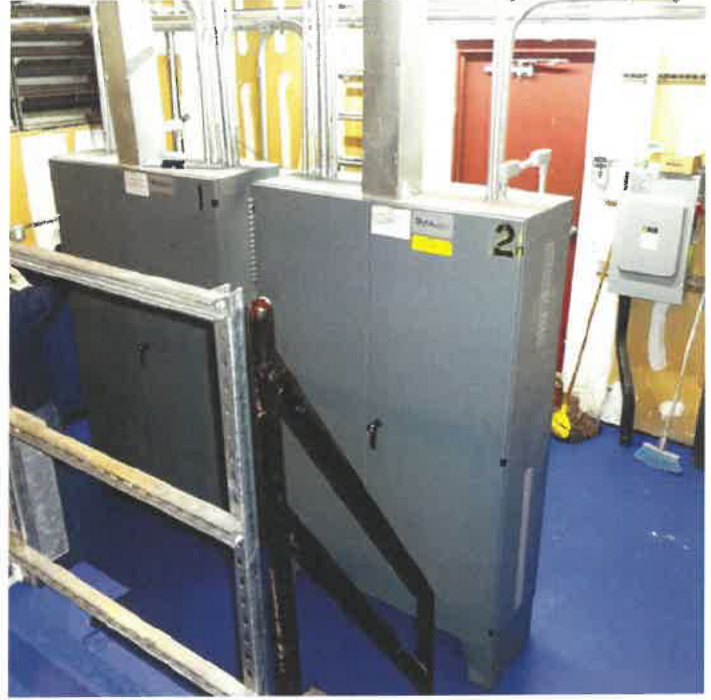
Machine Room After Modernization
