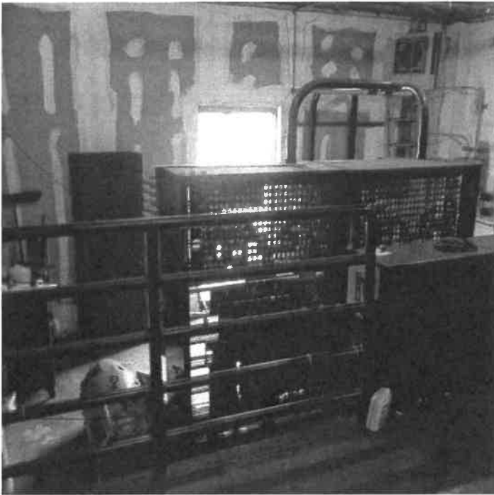
Machine Room Before Modernization
