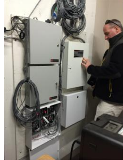
Frank Gallagher, Project Manager, conducts a site assessment on physical security infrastructure.
