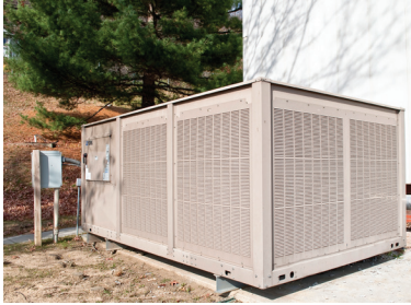
Bluefield State College - Generator
