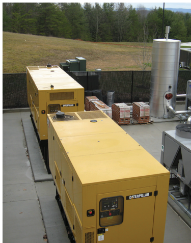
Alpha Natural Resources - New Headquarters Generators and Mechanical Units
