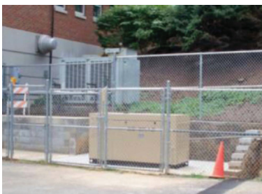
Radford University - Allen Building Electrical Generator
