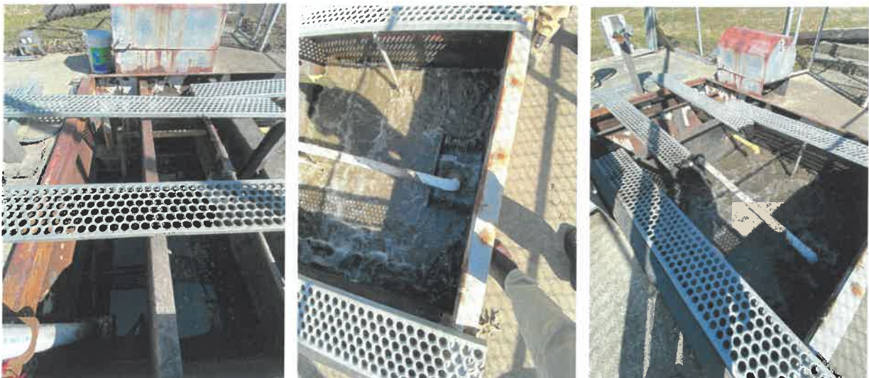
Views of the Barboursville School Package Wastewater Treatment Plant – photos by Dunn Engineers Inc.
