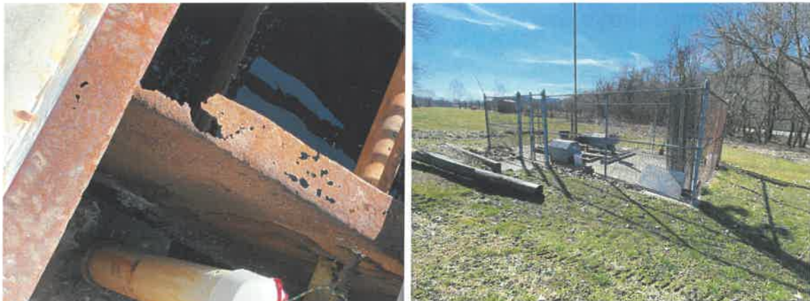
Above left, rust consuming metal parts of the 30-year-old package plant (above right). Photos by Dunn Engineers
