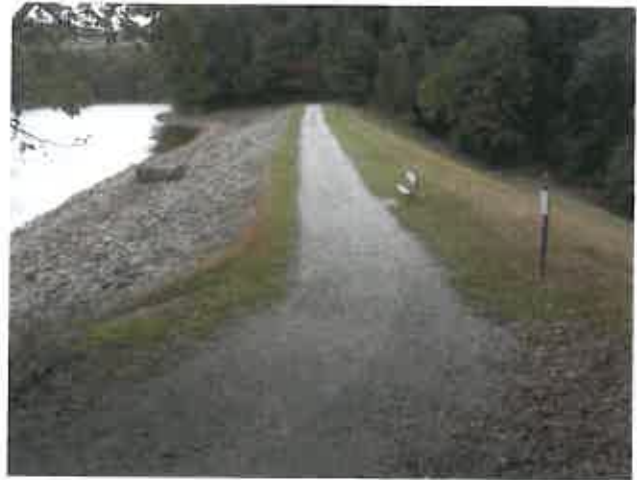
AECOM staff regularly visited the dam to inspect the overall condition of the embankment, principal spillway, slide gate, reservoir level, and remote instrumentation data collection system.
