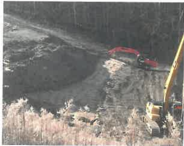
Drainage material and earthfill was placed and completed in accordance with the standard of practice for earth embankment dams.
