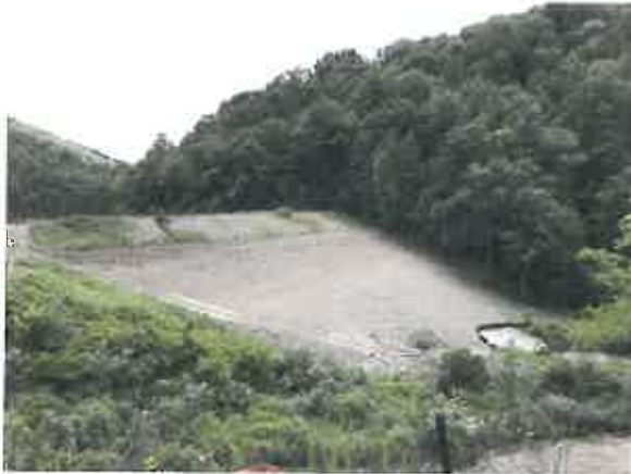
A blanket drain was installed on the downstream face of the dam to control seepage.
