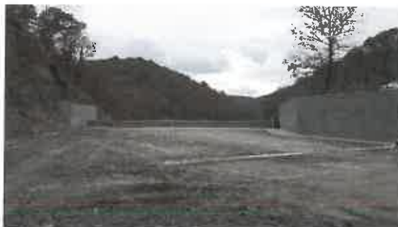
New spillway weir, new sidewalls to channel the flow over the weir and concrete cutoff trenches to improve the resistance of the bottom of the spillway chute to erosional forces.
