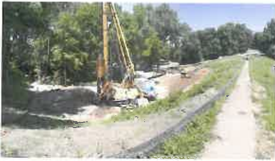
Liquefaction analysis resulted in the requirement for deep soil mixing to provide suitable liquefaction mitigation.
