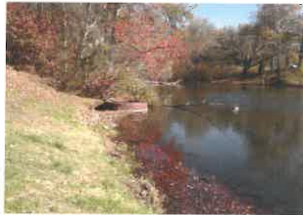
Existing principal spillway. To be modified into a new lake drain structure.
