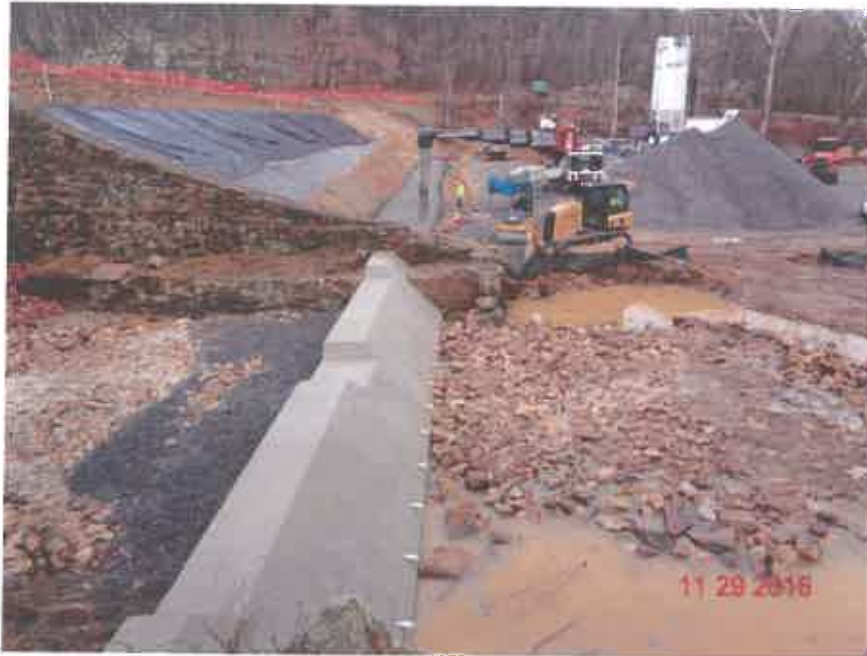
PARK DAM MODIFICATION (RCC PLACEMENT AND REINFORCED CONCRETE END DAM), CACAPON STATE PARK
