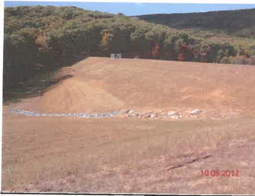
RESERVOIR DAM MODIFICATION, CACAPON STATE PARK (AFTER – NOTE BUTTRESS AT TOE TO CONTROL SEEPAGE AND IMPROVE STABILITY)
