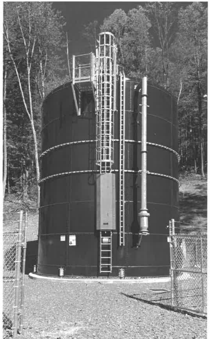
West Virginia American Water Project - Lewis County
