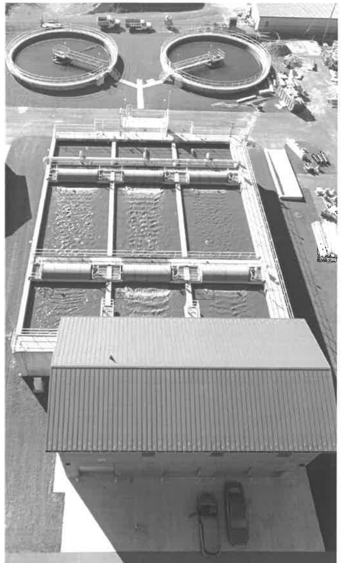
Vertical Loop Reactor System - White Sulphur Springs
