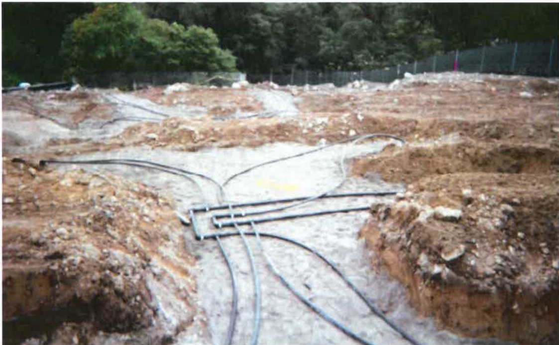
Typical Node (2) Manifold of Four 1.25" HDPE Pipes from Wells to 2" HDPE Header
