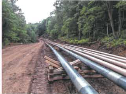
Natural Gas Pipeline Systems, Various Locations
