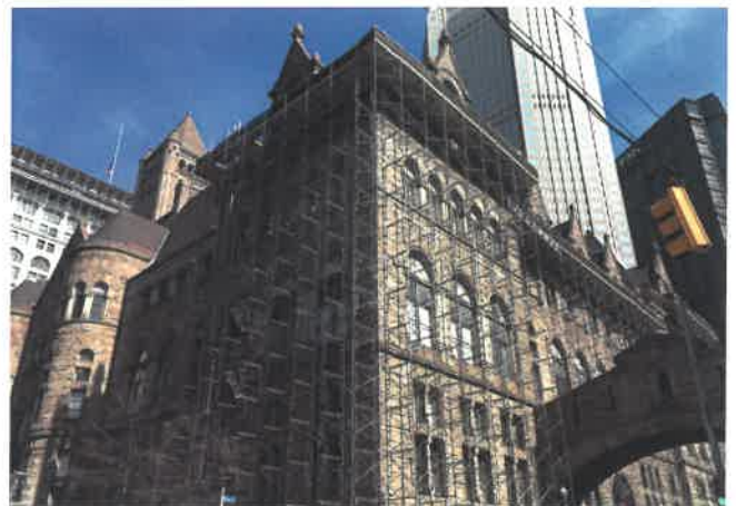
Construction under way, summer 2018—Scaffolding to the eave of the roof line; each week a crane is brought in to unload demo'd materials and load new tile to the top platform.
