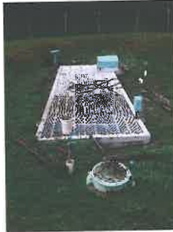
Original package treatment plant
