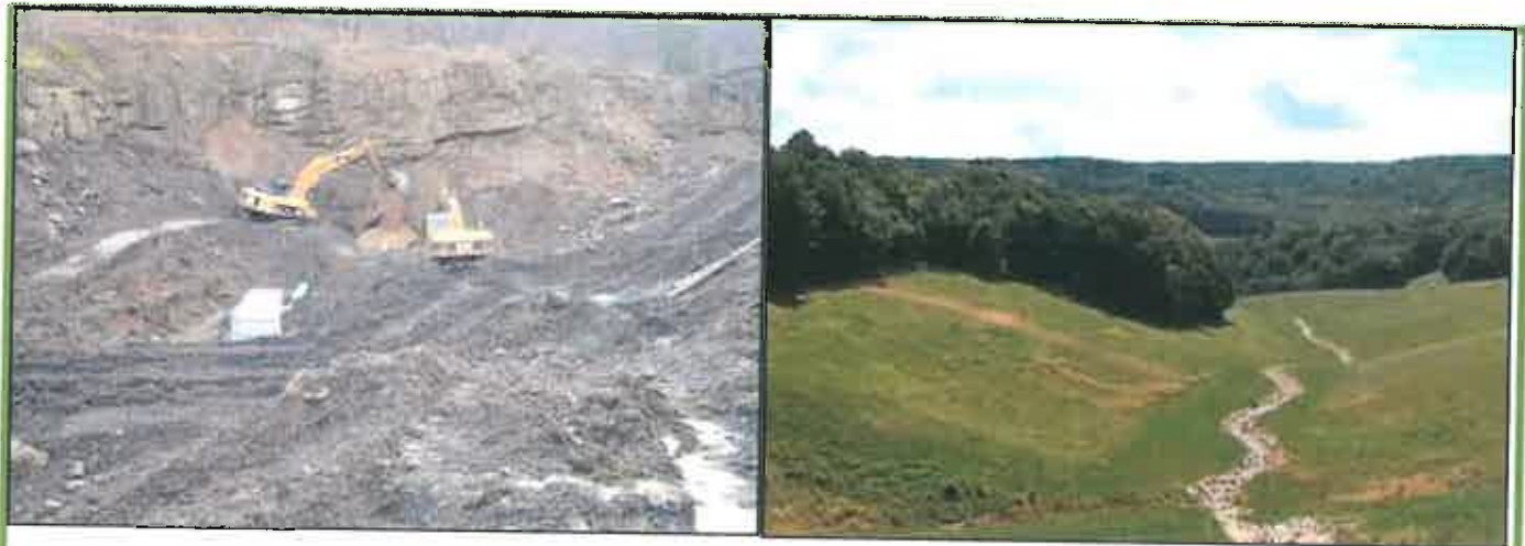
Kempton Refuse and Acid Mine Drainage/Abandoned Mine Lands Project in Tucker County, West Virginia. The West Virginia Department of Environmental Protection was honored by the U.S. Department of the Interior's Office of Surface Mining for its reclamation and restoration efforts on the Kempton Project. To find out more about West Virginia's Abandoned Mine Lands Program go to: http://www.dep.wv.gov/aml/Pages/default.aspx
