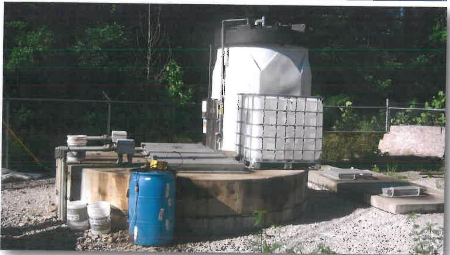
Boone County Public Service District—Calloden Pump Station with Odor Control Chemical Feed System
