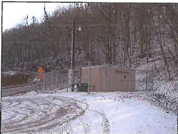
250 GPM Water Booster Station on Route 20
