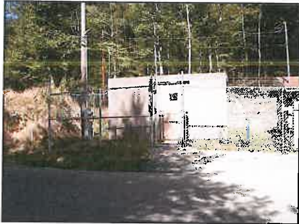
150 GPM Little Sand Run Booster Station
