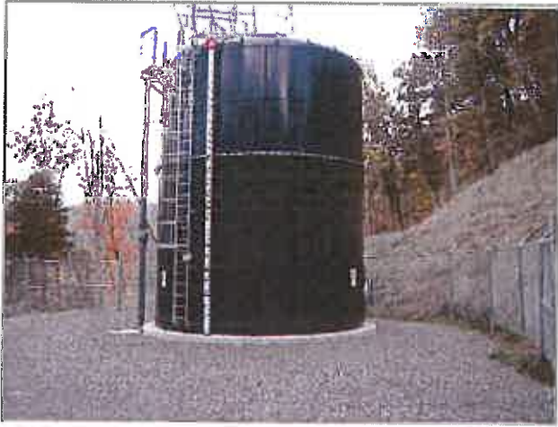
50,000 Gallon Storage Tank Near Mingo
