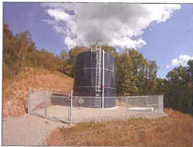
New 150,000 Gallon Water Storage Tank Above Whitmer
