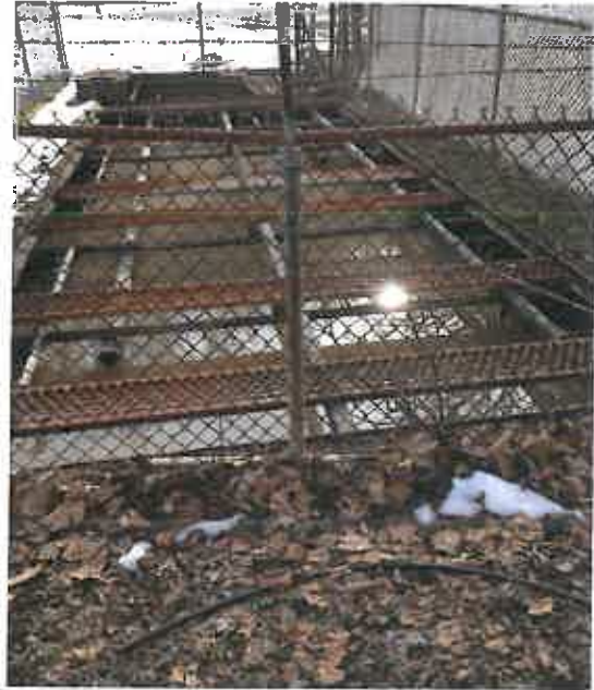
Failing Package Treatment Plant
