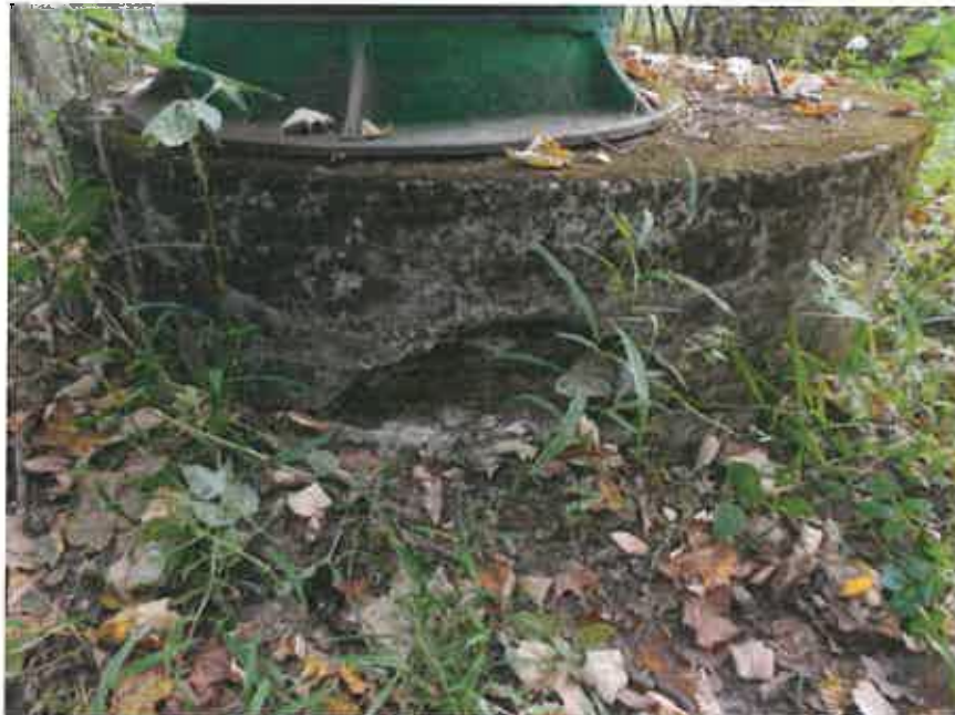
Manhole Identified for Replacement
