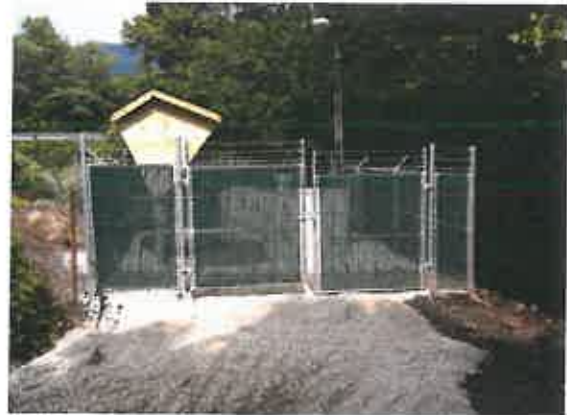
After: Upper Drive Lift Station
