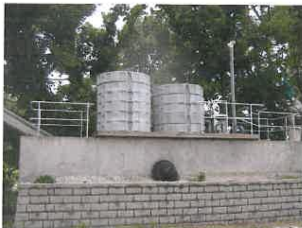
“Headworks” Facility with Scrubber Unit
