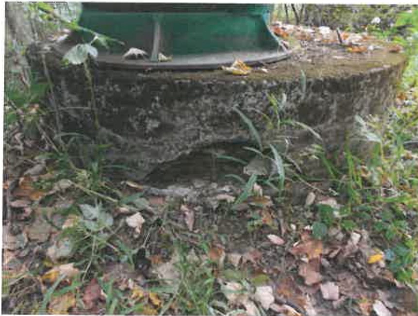
Manhole Identified for Replacement
