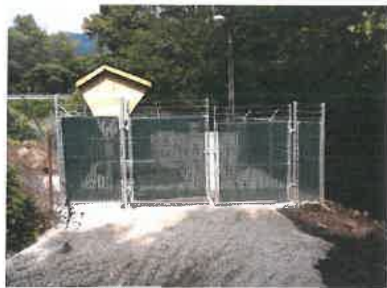
After: Upper Drive Lift Station
