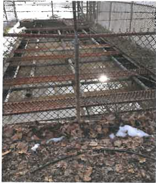
Failing Package Treatment Plant
