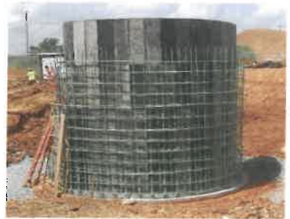
Charles Town Water Treatment Plant
