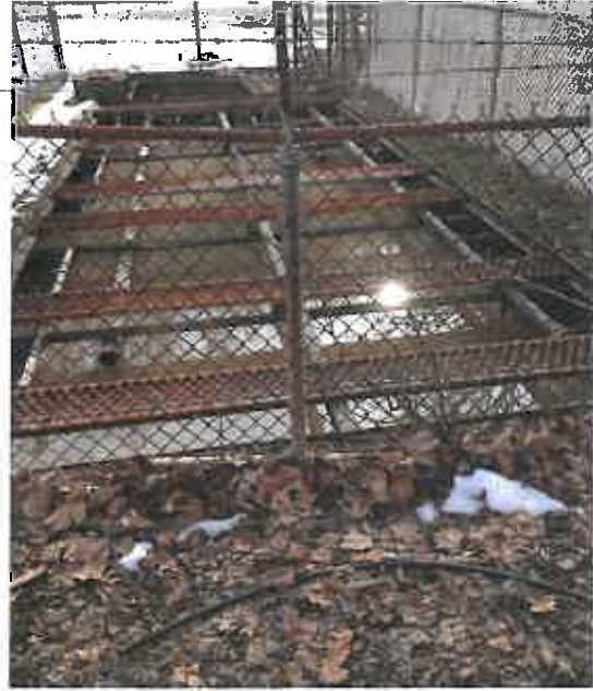
Failing Package Treatment Plant
