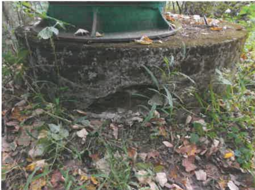
Manhole Identified for Replacement
