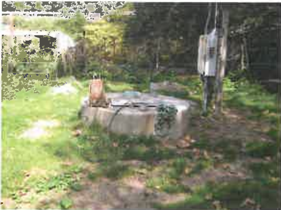
Before: Upper Drive Lift Station
