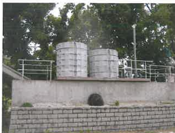
“Headworks” Facility with Scrubber Unit
