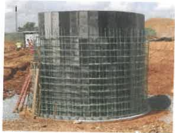
Charles Town Water Treatment Plant
