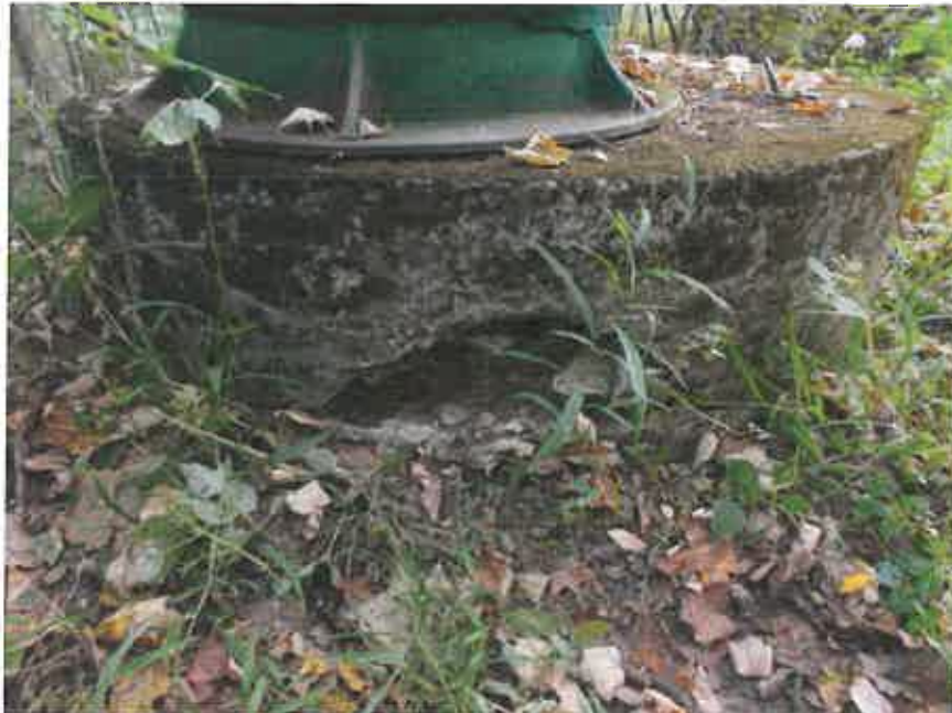
Manhole Identified for Replacement
