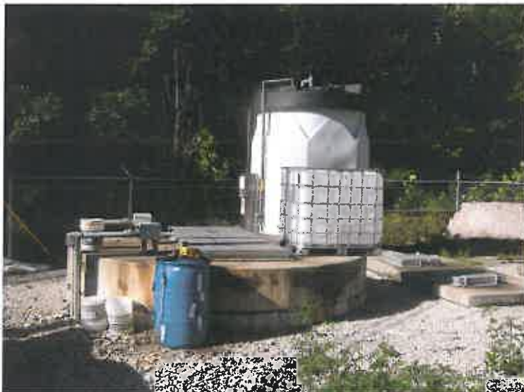
Culloden Pump Station with Odor Control Chemical Feed System in Background
