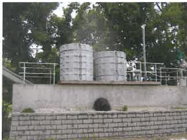
“Headworks” Facility with Scrubber Unit
