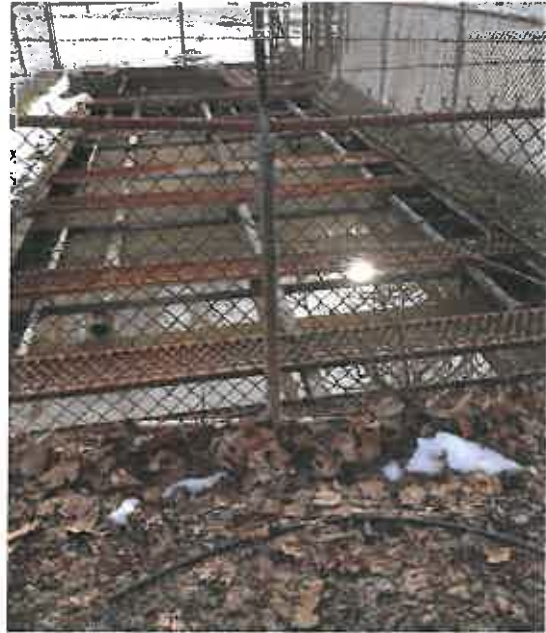
Failing Package Treatment Plant
