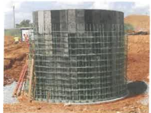
Charles Town Water Treatment Plant
